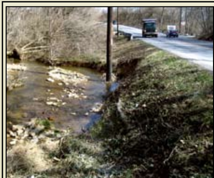
Who moved the pole? Streambank erosion can create problems for existing infrastructure.
