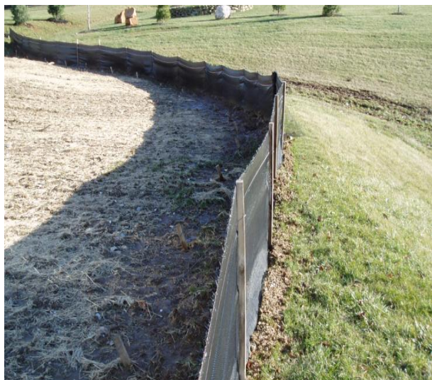
AN EXAMPLE OF FILTER FABRIC FENCE – This is a 30 inch reinforced fence.
