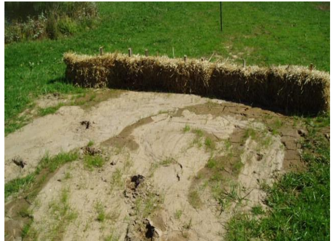
AN EXAMPLE OF STRAW BALES – Note the sediment accumulation upslope of the bales From Erosion and Sediment Pollution Control Program Manual, PADEP, March 2012 Courtesy of York County Conservation District
