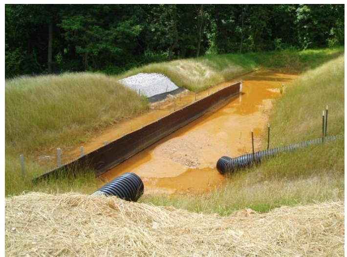
SEDIMENT TRAP - This sediment trap collects runoff from the disturbed site. Note the baffling to increase flow length. From Erosion and Sediment Pollution Control Program Manual, PADEP, March 2012 Courtesy of York County Conservation District
