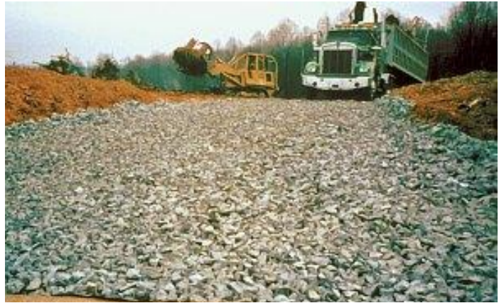
AN EXAMPLE OF ROCK CONSTRUCTION ENTRANCE - From Erosion and Sediment Pollution Control Program Manual, PADEP, March 2012 Courtesy Lake County Stormwater Management Department, Ohio
