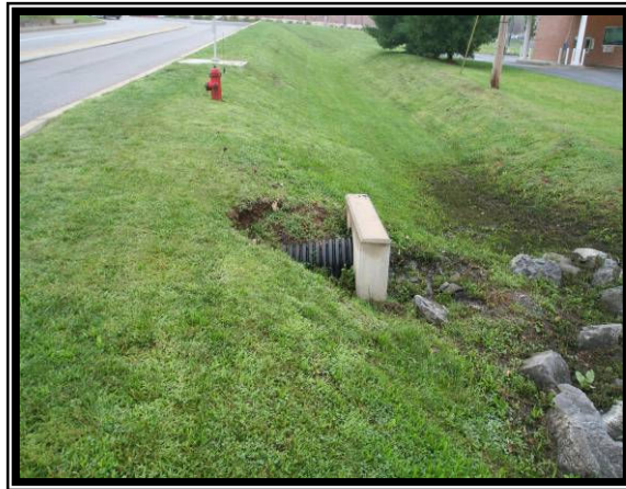
Photo 5 - Eroded endwall by Fulton Bank west of Cocoa Avenue
