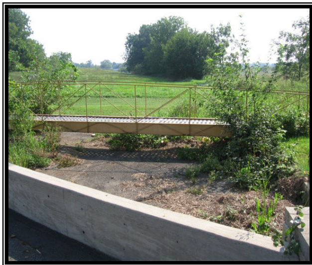
Photo 13 - The concrete wall that is supposed to protect the park from floods.
