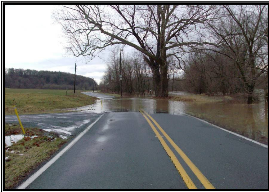
Photo 15 - Flooding at Bindnagle Road
