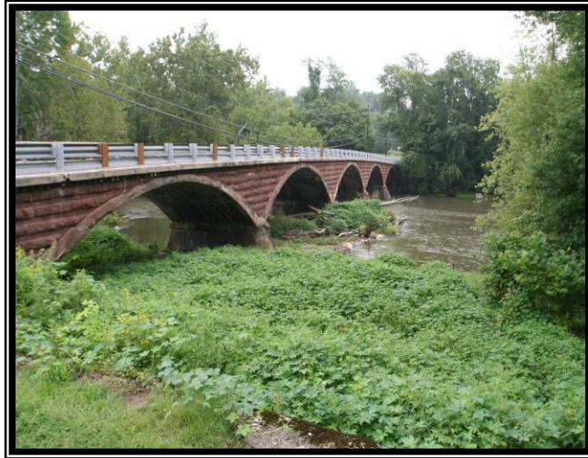
Photo 28 - Debris blocking the waterway opening of North Duke Street Bridge
