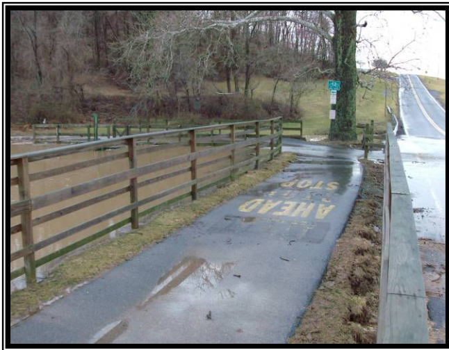
Photo 10 - Flooding of the Wood Road Pond
