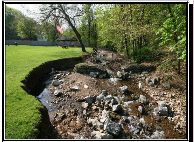
Photo 11 – Erosion at gabions upstream of pond
