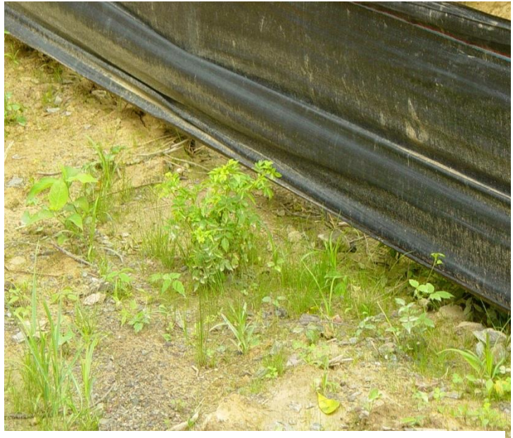
The silt fence below was not installed properly. It will not prevent sediment from reaching streams. Erosion control measures that are not installed properly waste your time and money.
