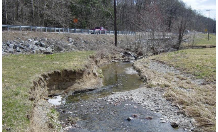
During storm events, unprotected streambanks allow soil erosion and deposition along Nyes Run.
